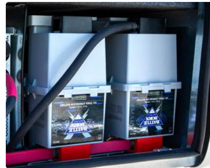
Additional Smart Lithium Battery 270-Ah 12-V with Internal Heating System (540-Ah total)
