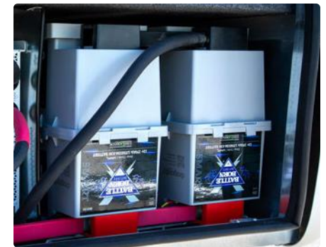
Additional Smart Lithium Battery 270-Ah 12-V with Internal Heating System (540-Ah total)
